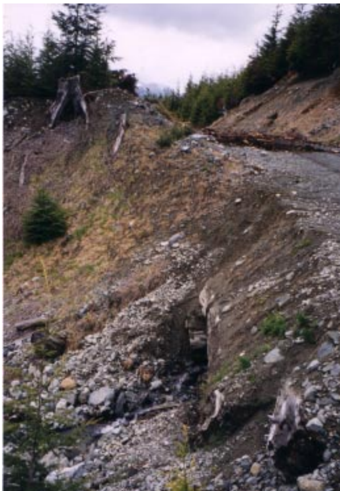
Figure 25. Evidence of rill erosion on the fill slope at Site 2.
