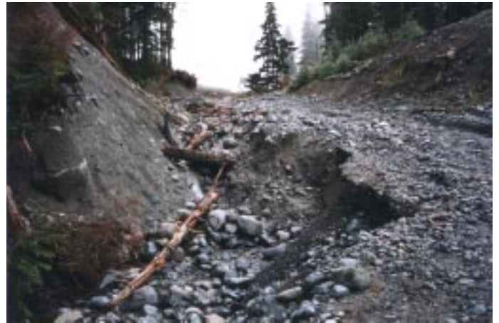
Figure 14a. Ditch above Site 45 after the washout of November 1995 and prior to road deactivation.
