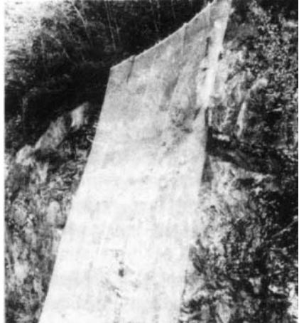
Mesh over an unstable slope
