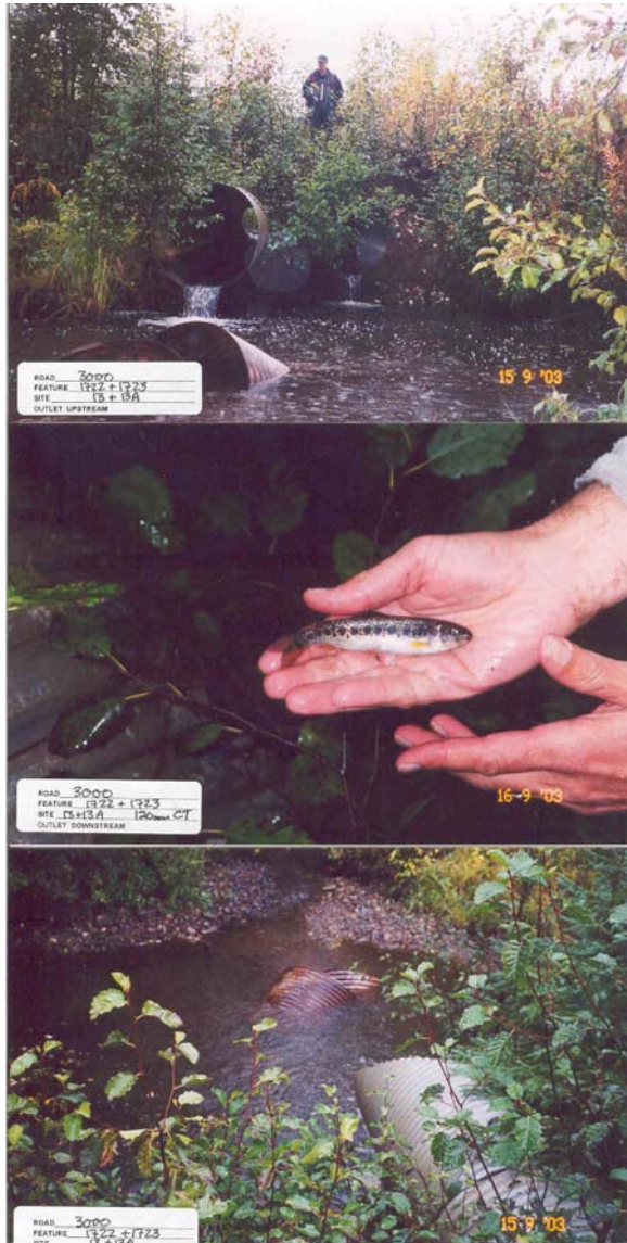
Photo 1. 3000 Road-Site 13/1722 culvert outlet conditions. 35cm outfall drop on both culverts.
