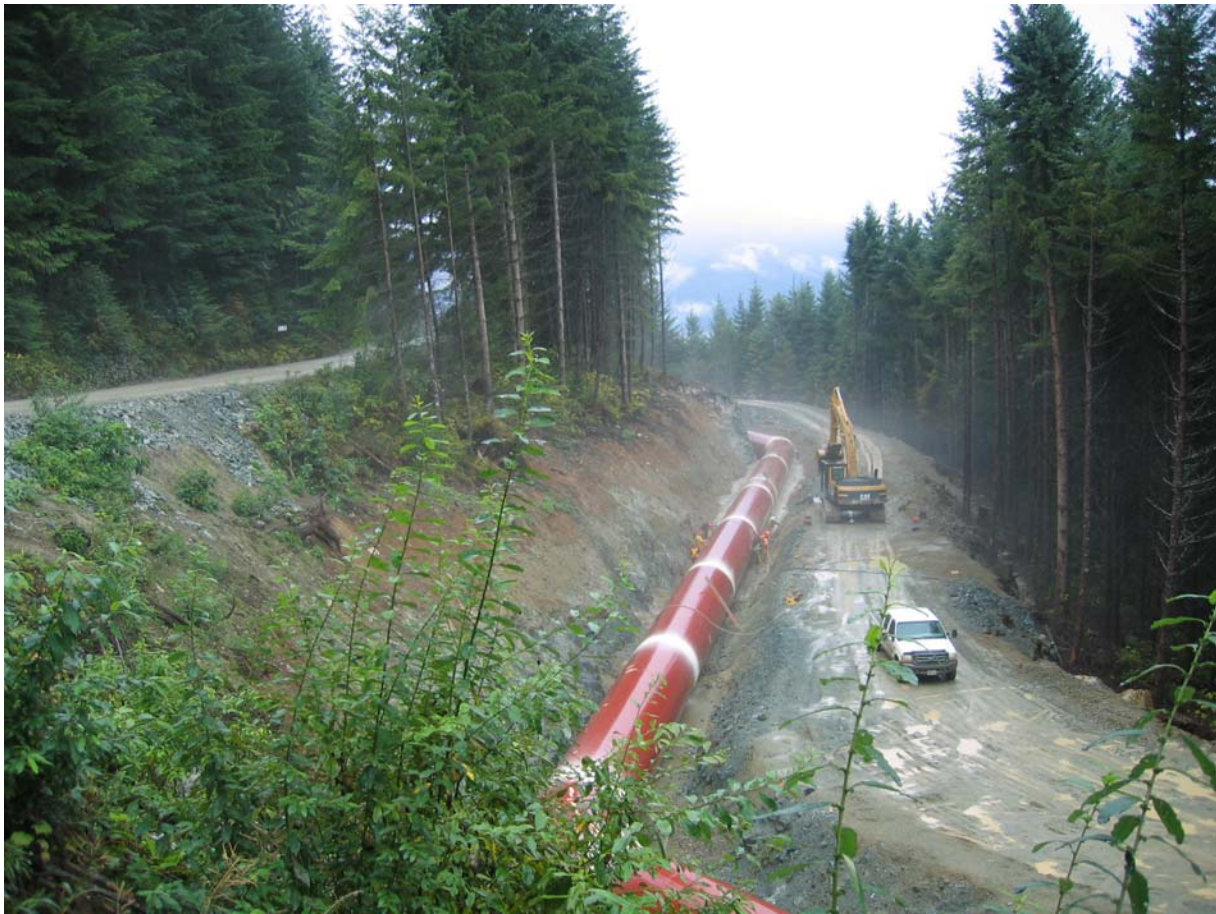
Upper Mamquam Waterpower Project, Squamish Forest District Penstock Pipe Installation Downhill of Mamquam Forest Service Road, September 2004
