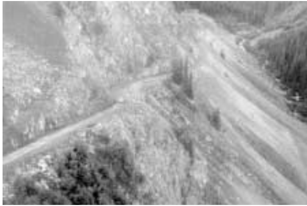
FIGURE 46 Looking south at the critical section of Option 4 following construction (C. VanBuskirk photo).
