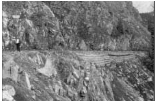
FIGURE 5 Roadfill supported by retaining walls to reduce the amount of full bench / end-haul necessary for construction of a forest road (C. VanBuskirk photos).
