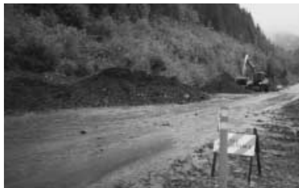
FIGURE 52 Debris being cleared from Highway 6, following June 4, 1999 debris flow (B. Ewings photo).
