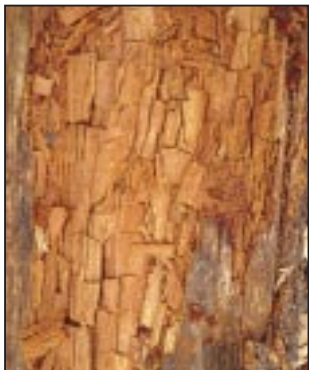
Brown rot – This cube-like type of wood decay is typical of most brown rot.
