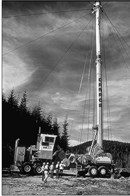
Figure 2 Large skyline towers can suspend logs over streams providing the conditions are suitable
