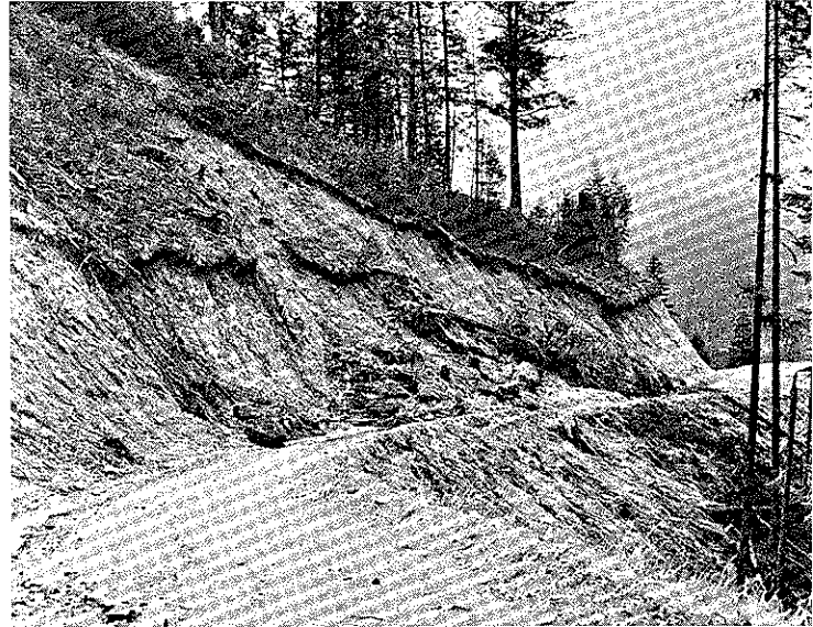
Figure 6b. Backslope failure along a logging road in the Salmon River Mountains of Idaho. Failure resulted from undercutting of the slope toe.
