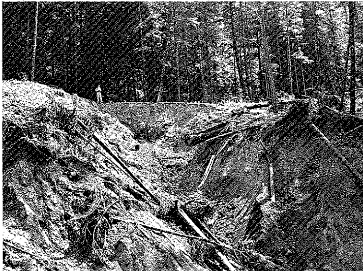
Figure 6c. Failure due to inadequate road drainage in the Cascade Range of Oregon.
