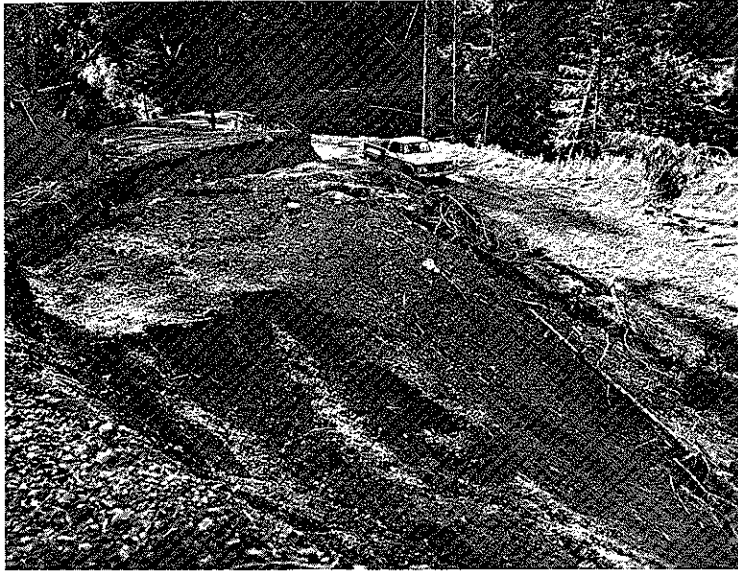
Figure 6. Examples of mass soil movements resulting from failure along a road right-of-way. a) Road fill failure in the Cascade Range of Oregon. Failure resulted from plugged side drainages and resultant saturation of the road prism.
