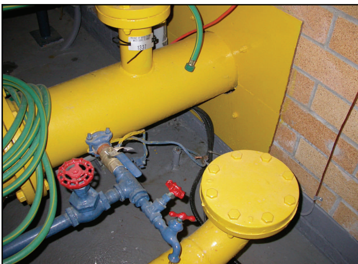
Plate 2. A picture of the raw water tap inside the Mackenzie pump house.
