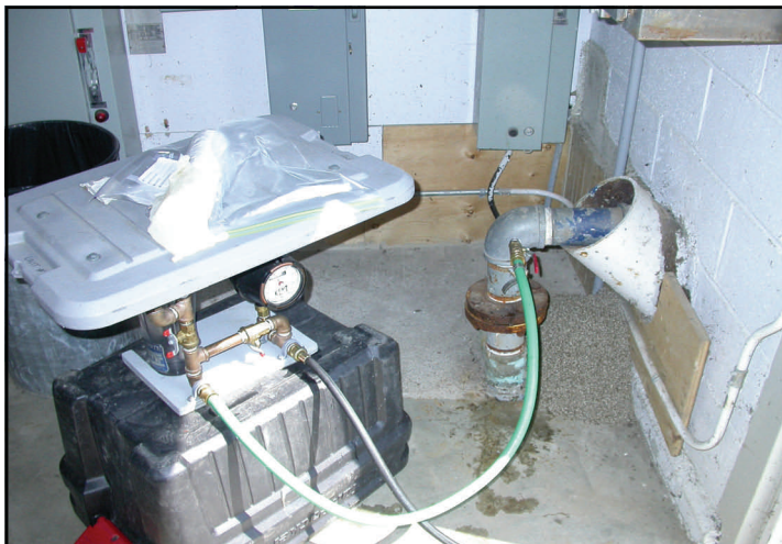
Plate 2. A view of the parasite kit beside the raw water tap in the Hudson's Hope pump house.
