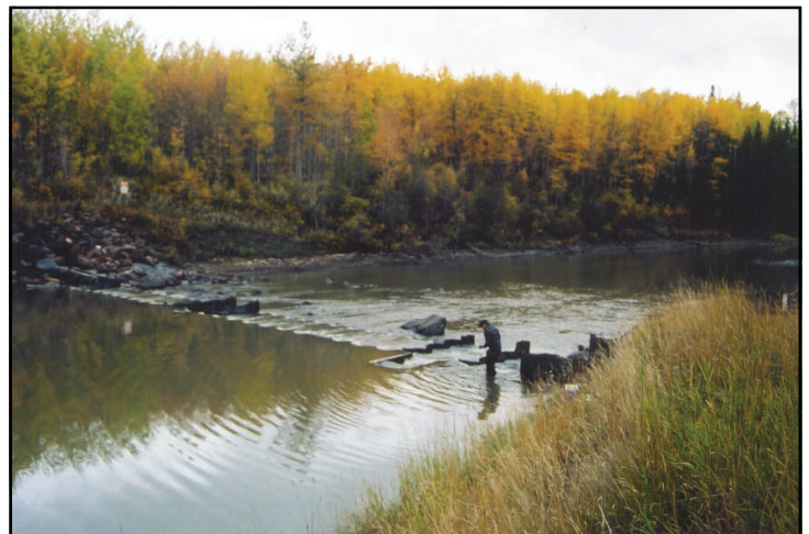
Plate 2. Cross-stream weir located immediately downstream of the Arras pump house. The weir raises water levels to ensure that there is sufficient water to support domestic users (October, 2002).
