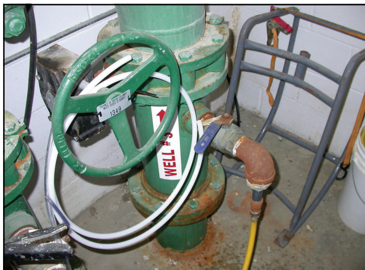
Plate 2. The raw water tap inside the Chetwynd pump house.
