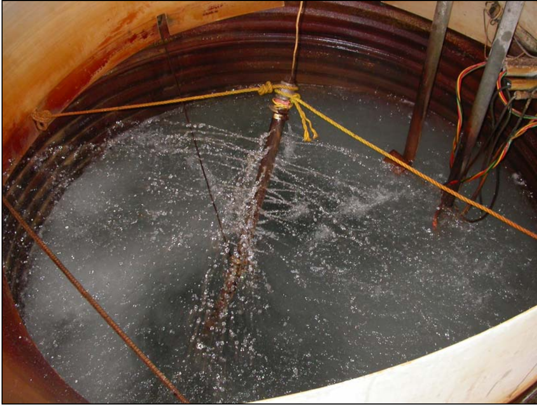
Figure 2. View of the Aspen Mobile Estates well aerator. The raw water is pumped up from the well and sprayed into this holding reservoir. A chlorine drip disinfects this water before it is distributed throughout the park. The red staining around the holding reservoir is from high iron levels in the water.
