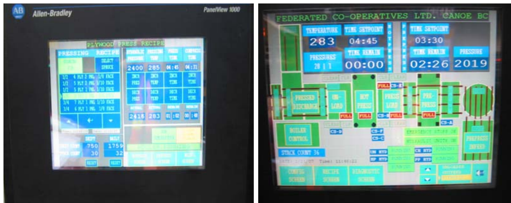
Figure 7: The pressing station interfaced with PLC and a Clouston compression control
