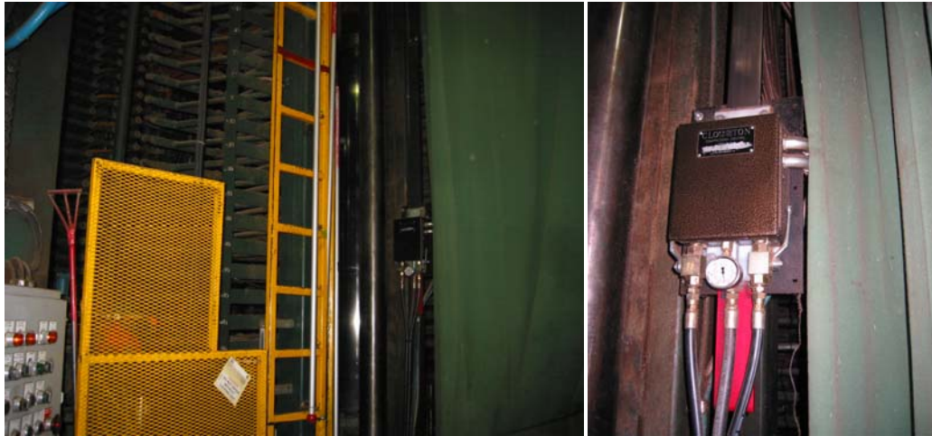
Figure 6: The 40-opening plywood hot press with a Clouston compression control
